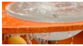
Water Damage Baltimore
