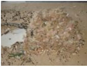
Baton Rouge Air Duct Cleaning
