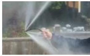
drain cleaning service
