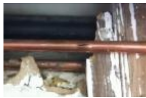
Frozen Pipe Burst
